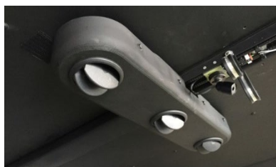
Figure 2-16. Air Conditioning Vents.
